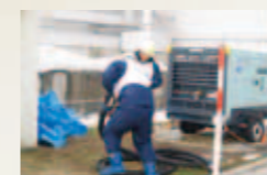
エンジン付き空気コンプレッサーの接続訓練 Training in connecting a hose to an air compressor with an engine
